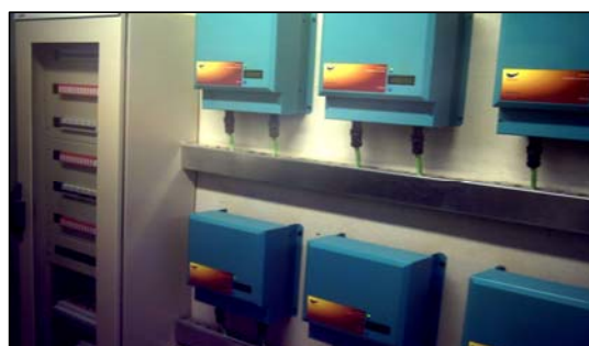
SINEO-3K3 IN EQUIPMENT ROOM
